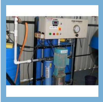
RO Water Treatment Plant
