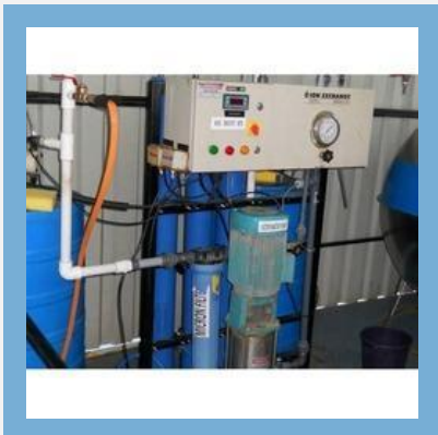
Drinking Water Treatment Plant
