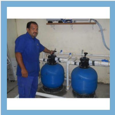
Swimming Pool Filtration Plant
